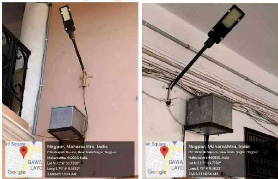
Solar Lights installed in campus and corridors
