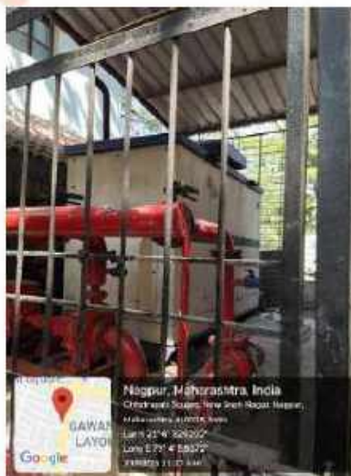
Diesel Generator in college
