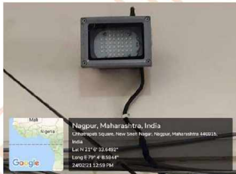
Solar Lights installed in office
