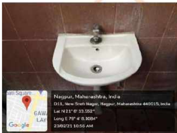
Taps to be replaced by Faucets
