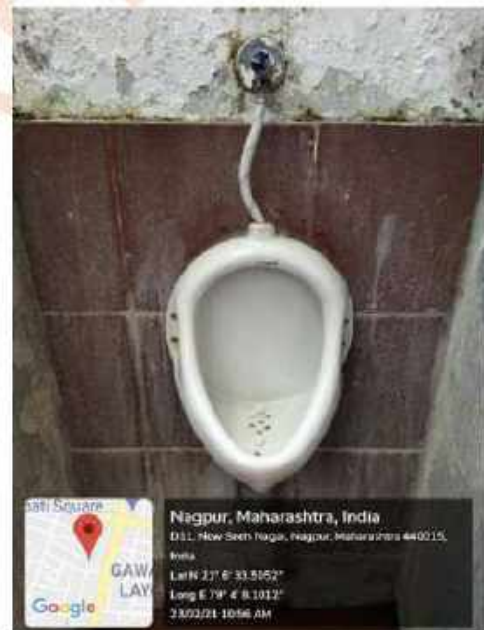
Flush to be replaced by Push Buttons
