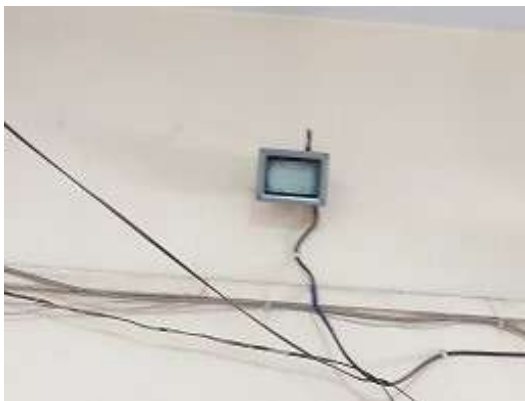
Solar Light Used In Office
