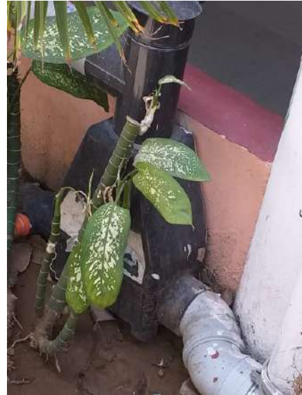
Rain Water Harvesting Valve
