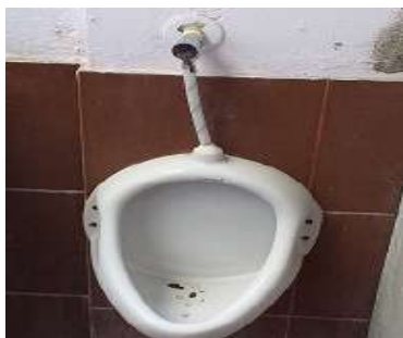
Toilets with simple taps
