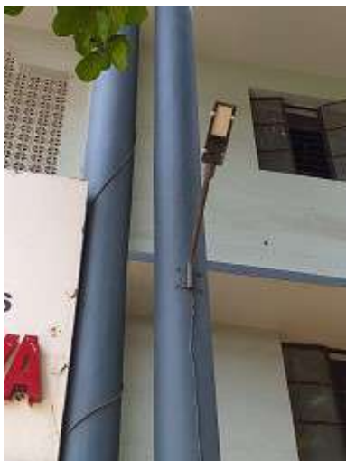
Solar Light Used In Campus
