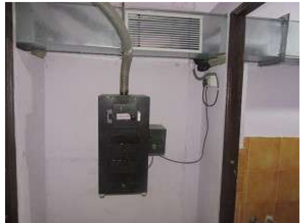
Incinerator machine for disposal of sanitary waste
