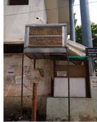
Cooler used for Office cooling
