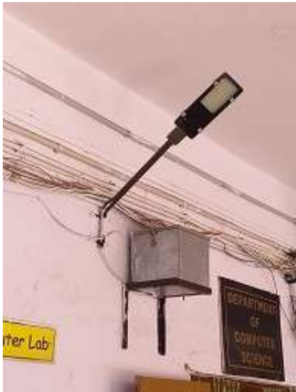
Solar Light Used In Corridors
