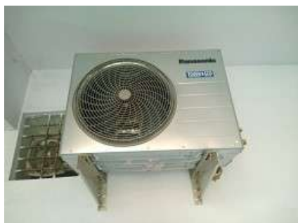
Condensers installed in Shade that reduces condenser pressure and hence compressor works
