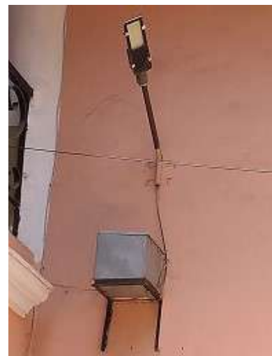
Solar Light Used In Campus
