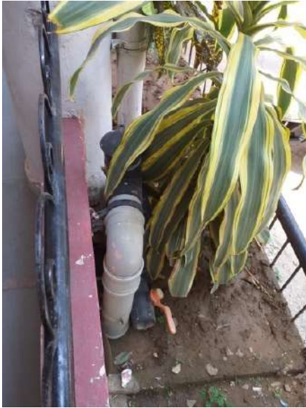
Rain Water Harvesting system
