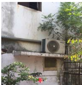
Placing the Condenser in shade reduces condenser pressure and hence compressor work
